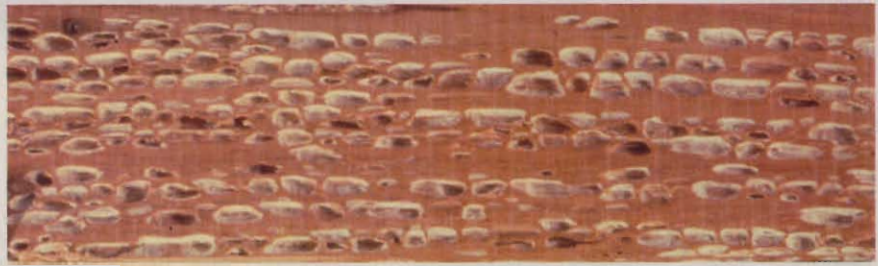
Staining fungi (closeup)
